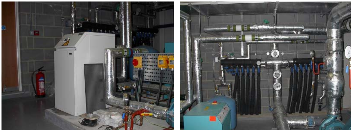
Figure 11. Commissioning (plantroom with heatpump and manifolds): demarcation of the groundsource at the manifold.
